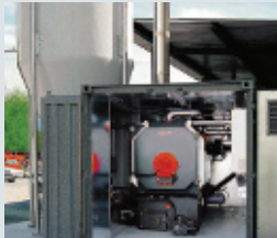
Viessmann Production Plant Wolfurt, Austria
